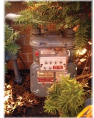
A meter means you'll find an underground line in the area.
