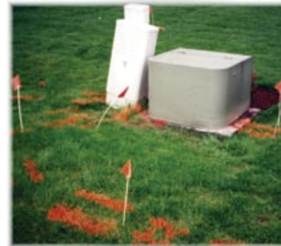
Pedestals near your work site are an indication that underground lines are in the area.
